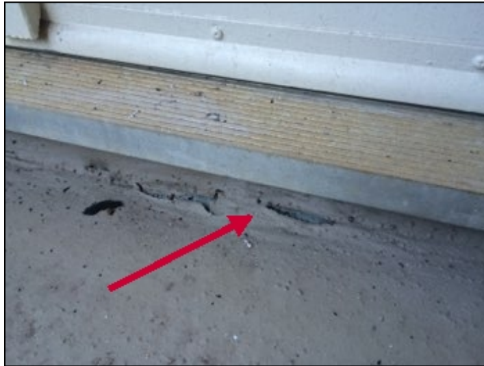
Damaged waterproof deck coating at master bedroom lanai.
