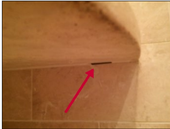
Missing grout under seat at master bathroom shower.
