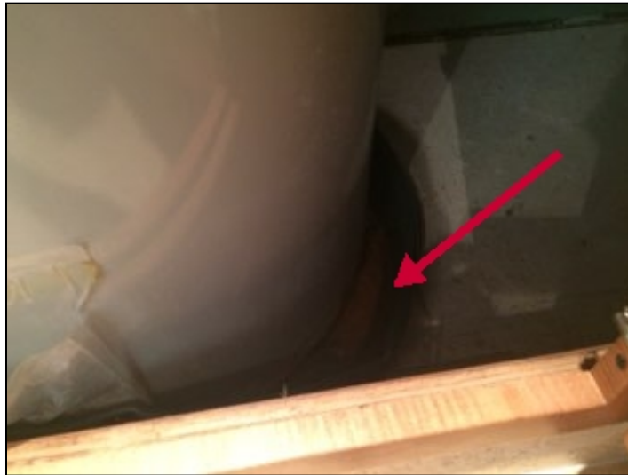
Corrosion, water in pan at water heater.
