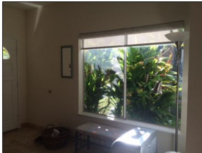
Dining room window difficult to operate.
