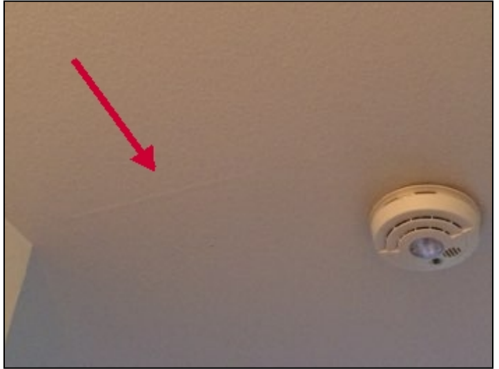
Master bedroom ceiling defect.
