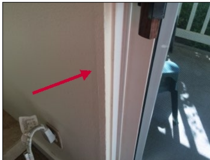
Minor drywall damage at living room lanai.
